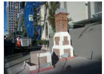
Canterbury Club, Christchurch, 2012 replacement with single wythe brick over steel frame . Photo, Heritage New Zealand
